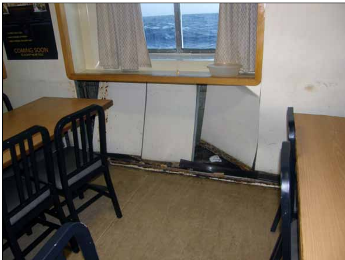
Damage to crew mess room, Deck 3
